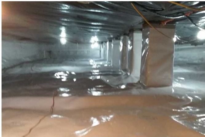
The photo above shows the completed crawl space repairs with the moisture control products in place that will keep the crawl space clean and dry.
